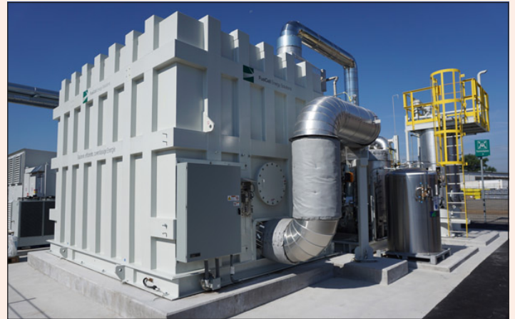
The 1.4 megawatt fuel cell is expected to provide around 60% of the energy required for FRIATEC's production processes.
